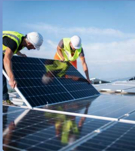
Rooftop PV solar panels saves on energy consumption.
